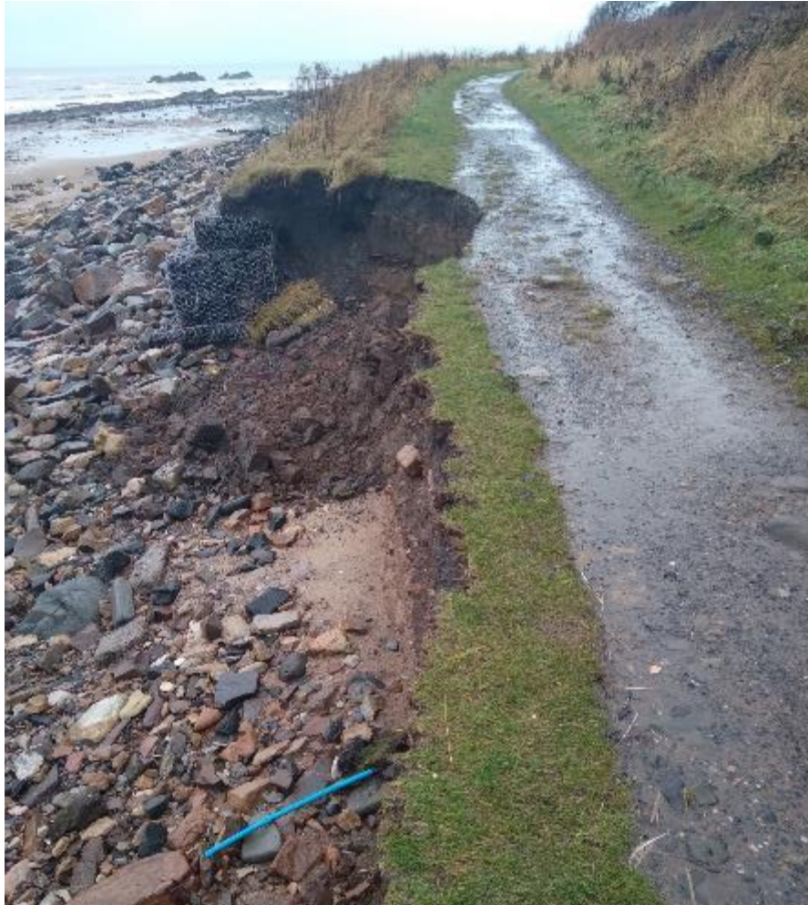
Seafield – Coastal Path Damaged
