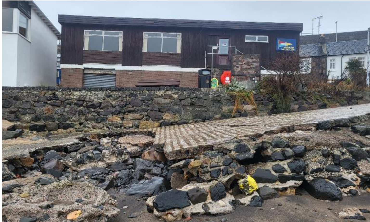
Kinghorn – Slipway Damaged
